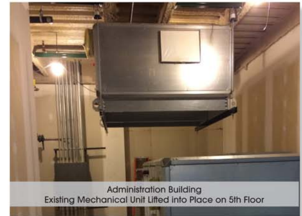
Administration Building Overhead Mechanical and Electrical on 5th Floor
